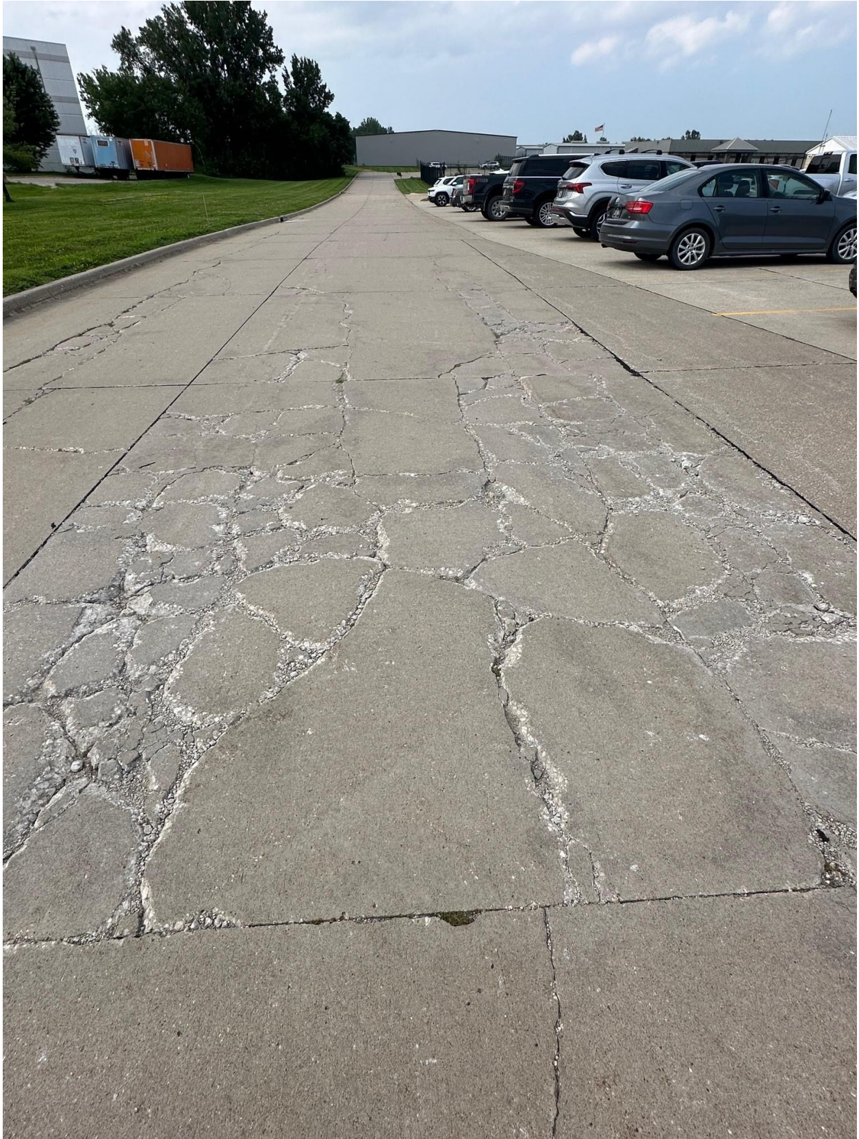
Figure 4: Entrance Road Condition
