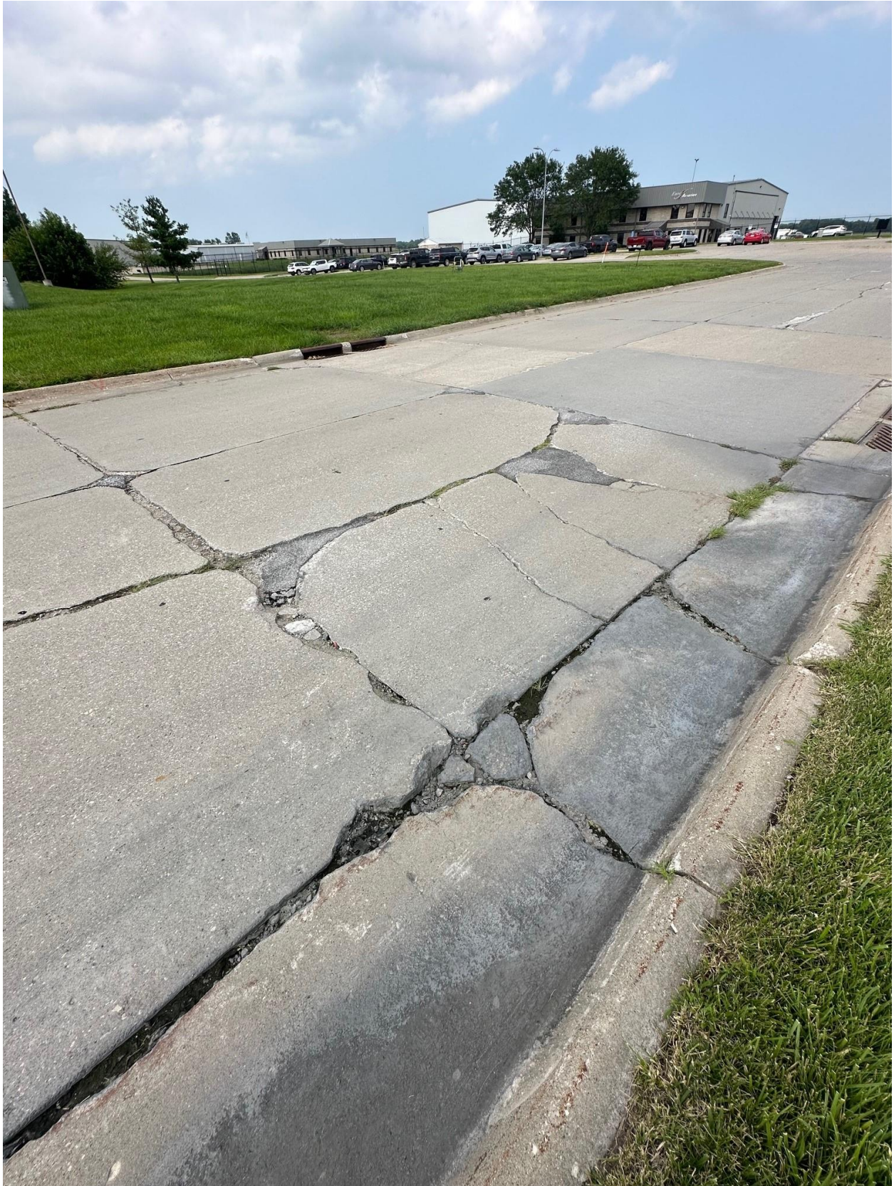
Figure 3: Entrance Road Condition
