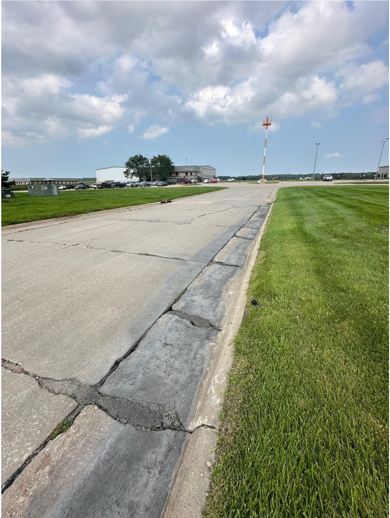
Figure 2: Entrance Road Condition
